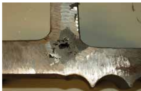
Abb. 09-1 Lunker in GJS
