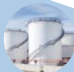
Corrosion detection of storage tanks
